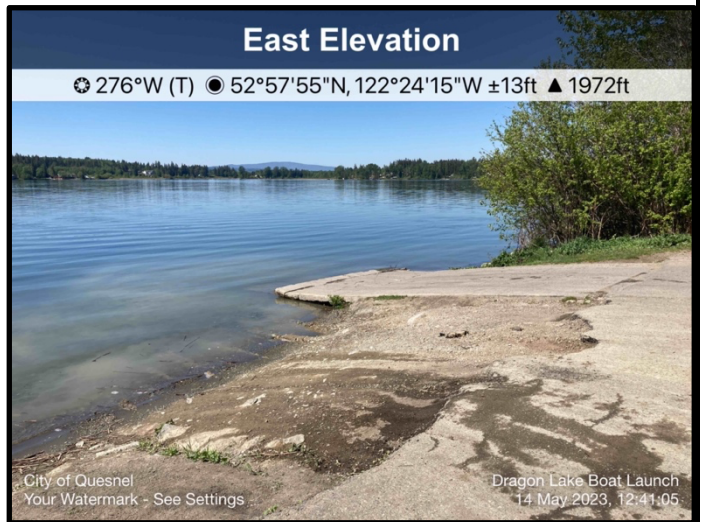
Access May 14 th 2023: Damage to Area Adjacent to Boat Launch Structure
