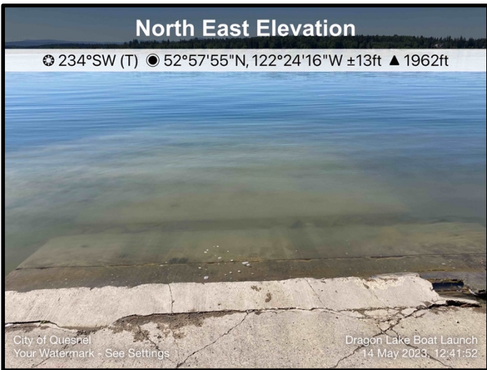
Access May 14 th 2023: Damage to Existing Boat Launch Structure
