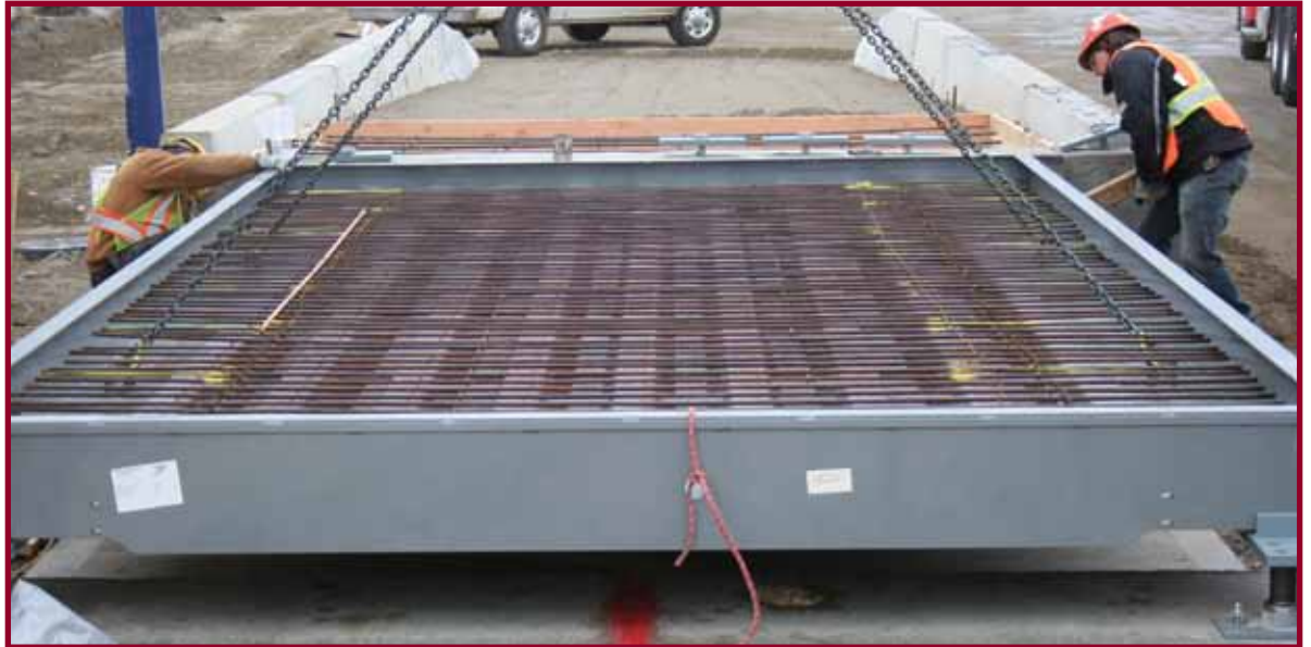
Crews install one of the new scale decks at the Quesnel Regional Landfill. The new system is designed to divert waste from the landfill, reducing future costs and the negative environmental impacts.
