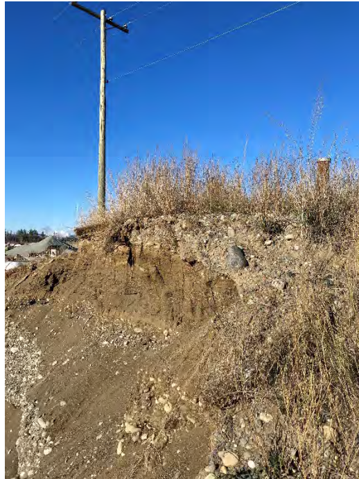
PHOTOGRAPH 7: Undercutting of area below access to MW11-13D and MW11-13S.
