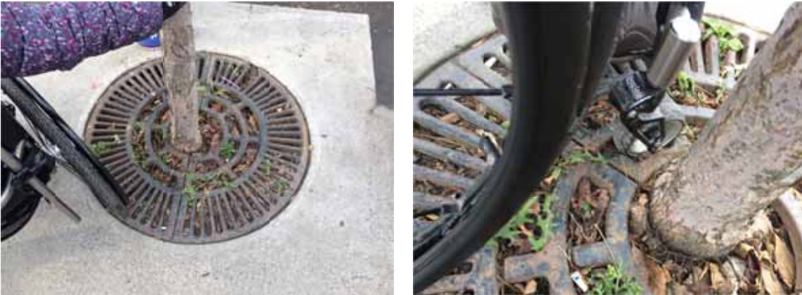
Photo 34: Tree grate openings are too large and are a hazard for mobility devices
