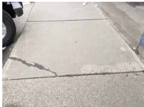
Photo 113: Cracked concrete by Quesnel Chiropractic
