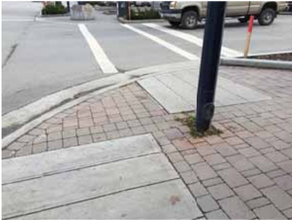
Photo 66: NW corner of Reid St. and St. Laurent Ave with pole that obstructs view
