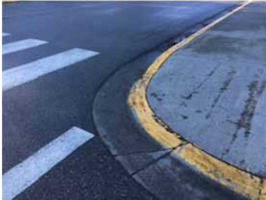
Photo 202: Jones Street and St. Laurent intersection – curb at NW corner
