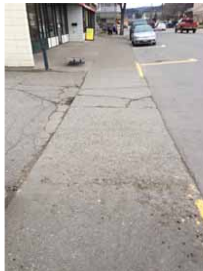
Photo 211: Cracked pavement by alley
