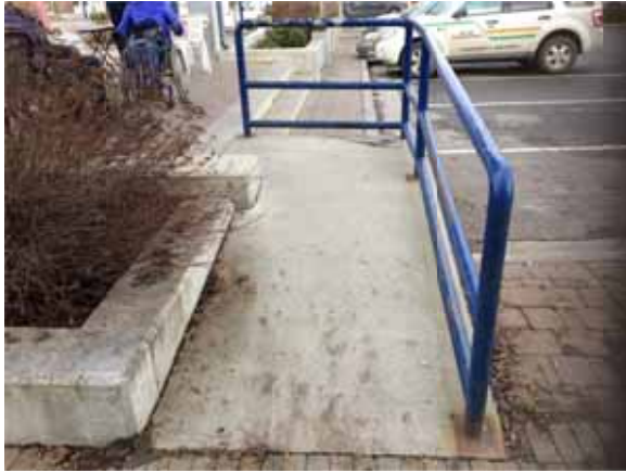
Photo 73: Ramp provides access to raised area but limited space for people using larger mobility devices (only 1 m wide at its narrowest section)
