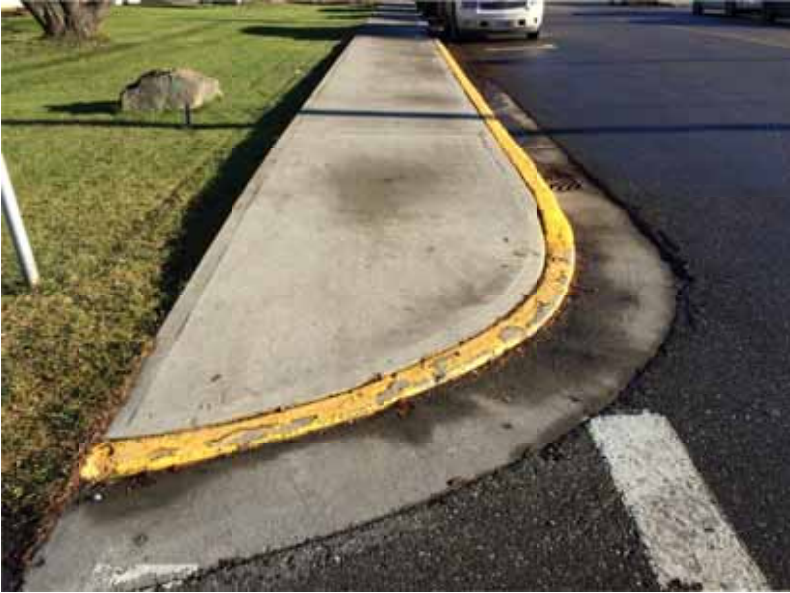
Photo 207: NE corner of Jones St and St. Laurent Ave – lip/dip at transition between curb and street & lacks tactile warnings
