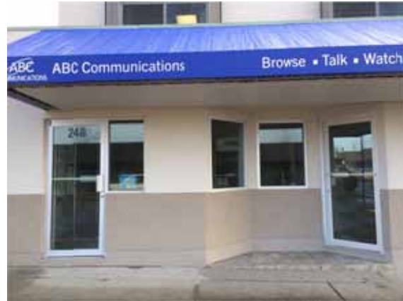
Photo 118: Abrupt change in elevation in front of ABC Communications
