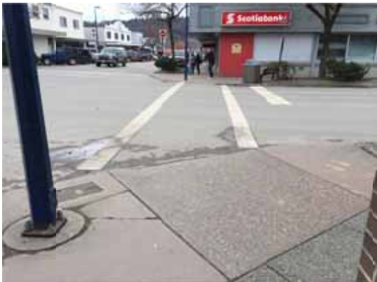
Photo 91: NW corner of Reid St. and Barlow Ave looking south – Areas with cracked concrete
