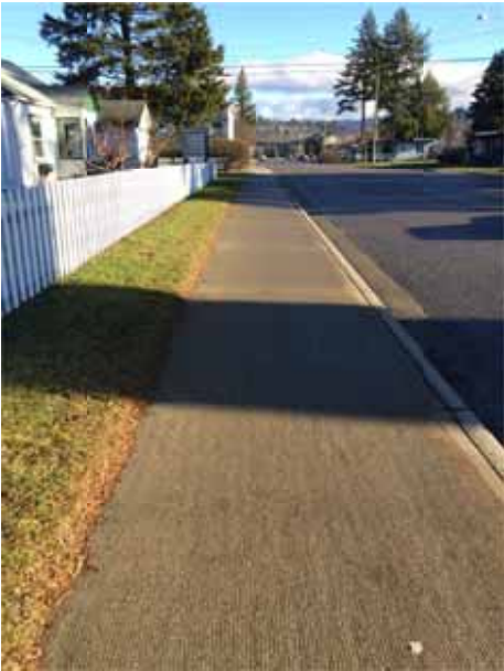
Photo 188: Heading east along St. Laurent on the north side of the street – Good new crosswalk between Callanan St and Wilson St with smooth transitions
