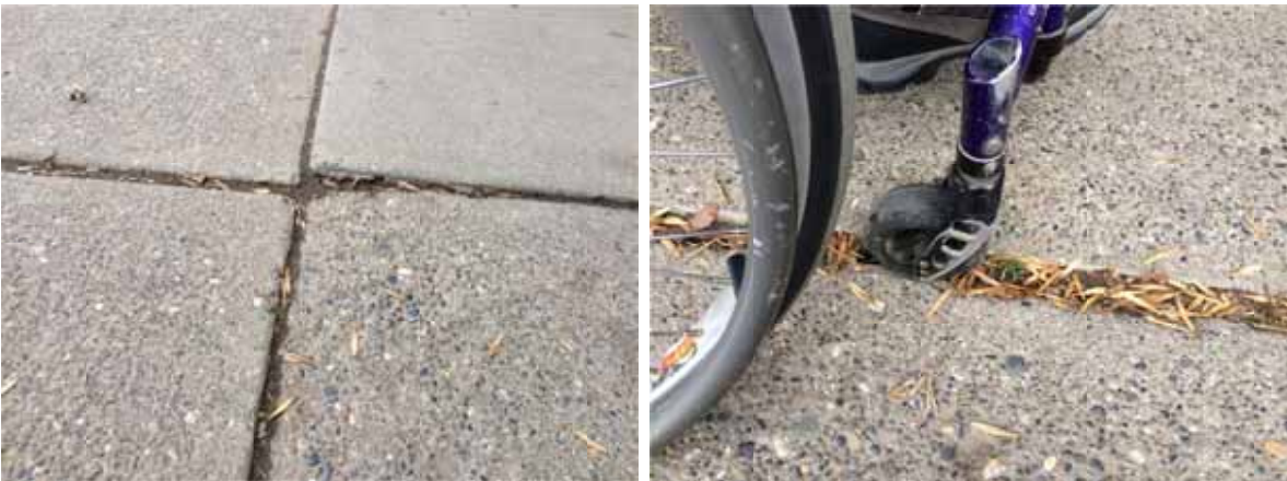
Photo 33: Older sections of sidewalks have large gaps in between concrete sections (sometimes as wide as 38 mm) – these are a hazard for people using mobility devices
