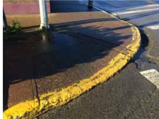
Photo 126: SW corner of Reid St and Carson Ave lacks proper curb ramp
