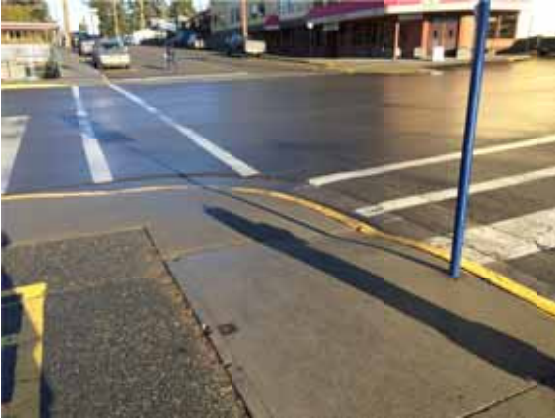
Photo 43: SW corner of Shepherd Ave and Reid St looking NE towards Begbies – Gaps in the transition between the curb ramp and roadway
