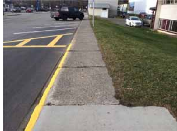
Photo 25: Sidewalk narrows along Shepherd Ave (west of Reid St) to 1120 mm which is not enough space for two people in mobility devices to pass by each other in opposite directions
