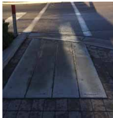
Photo 158: Looking north from the SW corner of Kinchant St and St. Laurent (curb with tactile lines)
