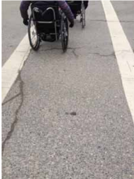
Photo 219: Crossing Barlow Ave from the Casino towards the Provincial Office – Cracked pavement
