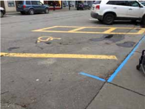
Photo 78: Accessible parking spot in front of CIBC
