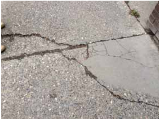
Photo 50: Cracked pavement in front of Reason to Run
