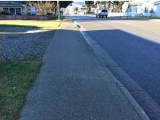
Photo 190: Heading westward on south side of street – Cross slopes
