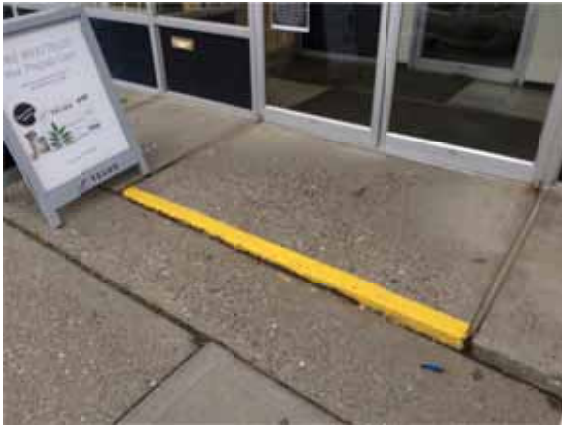
Photo 117: Abrupt change in elevation in front of Telus Store
