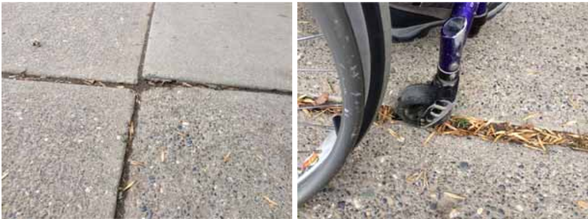
Photo 48: Older sections of sidewalk have large gaps in between concrete sections that are a hazard for people using mobility devices (sometimes as wide as 38 mm)
