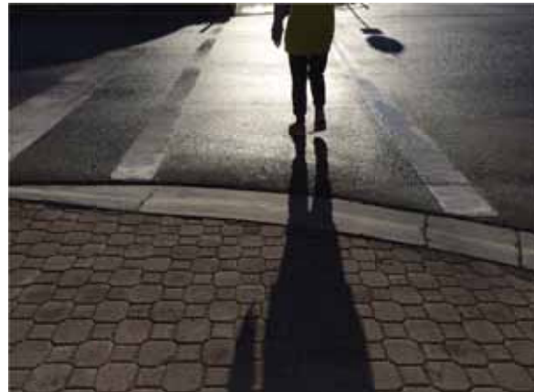
Photo 154: Curb ramps lack tactile/visual guides for people with visual disabilities
