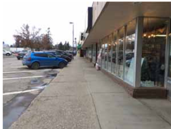
Photo 49: Puddles form along Reid St—will create an icy, slippery road surface in winter
