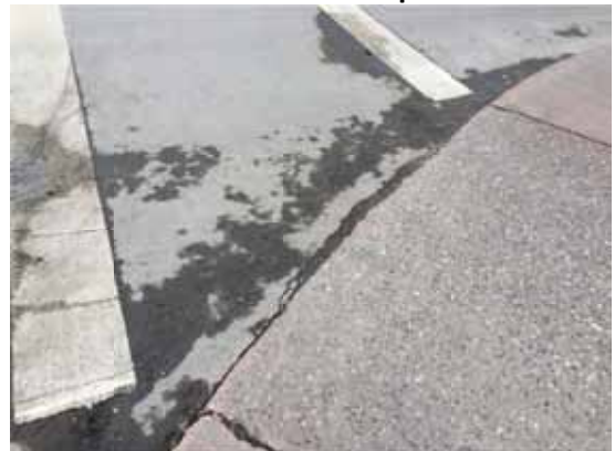
Photo 92: NW corner of Reid St. and Barlow Ave looking east – Cracked concrete at transition between curb ramp and crosswalk
