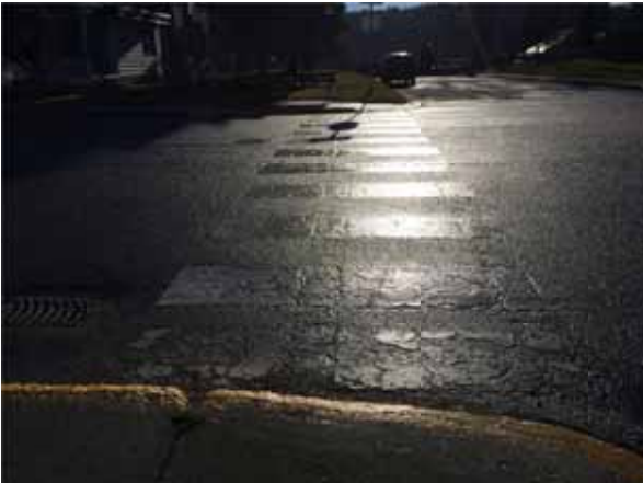
Photo 195: Extend painted yellow area to provide enough space for bus
