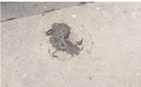
Photo 104: Freeze thaw action caused cracked pavement where pole was removed.
