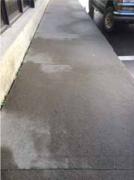
Photo 30: New section of concrete sidewalk on Barlow Street by TD Bank with smooth transitions between different sections of concrete
