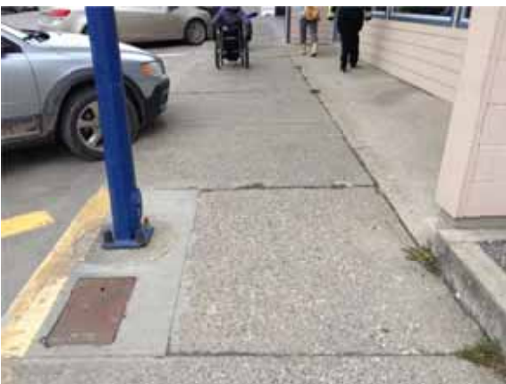
Photo 112: Cracked concrete in front of Autoplan Insurance
