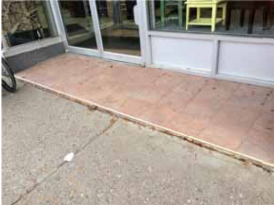
Photo 75: Uneven transition between City sidewalk and area in front of City Furniture creates barrier for mobility devices.
