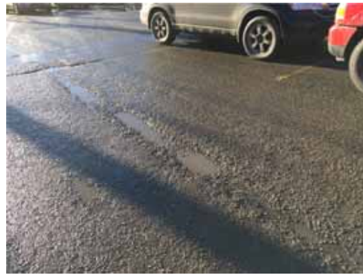
Photo 132: Broken pavement and puddles in alley
