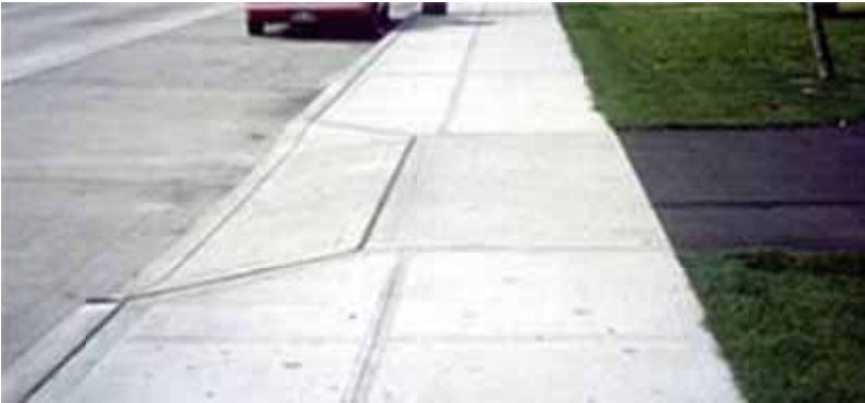
Photo 27: Example of driveway curb ramp where it does not impede the path of travel (min 915 mm)
