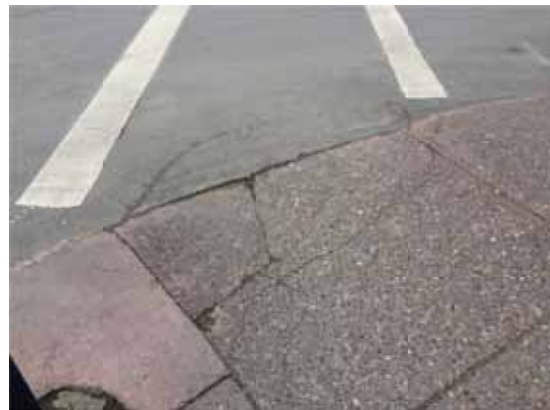
Photo 97: NE corner of Reid St. and Barlow Ave looking west – Cracked concrete
