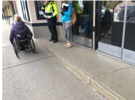
Photo 87: Step leading up to Movie Theatre is a potential hazard that is not well marked
