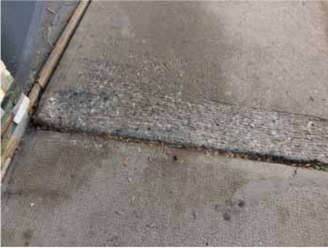
Photo 114: Cracked and rough pavement by Willis Harper
