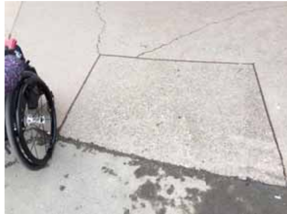
Photo 94: Cracked concrete at SW corner
