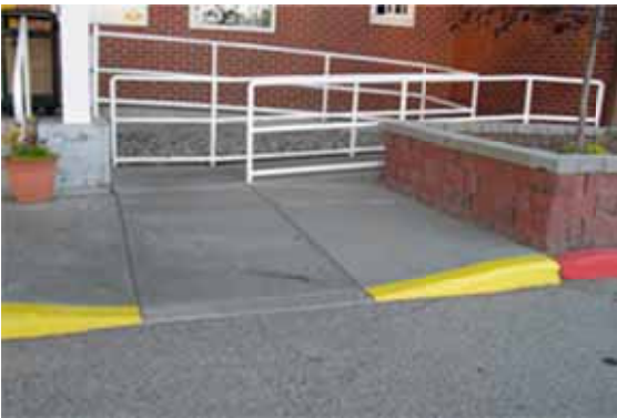
Photo 28: Example of using paint to warn people with visual disabilities about the presence of a curb ramp 4
