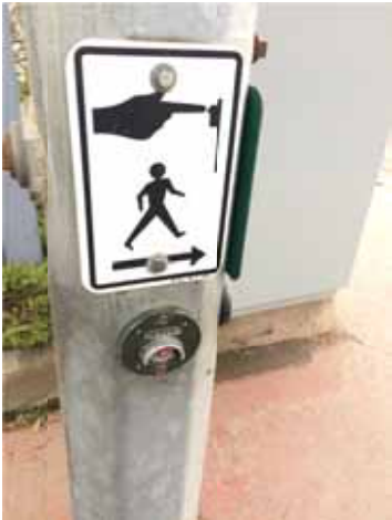
Photo 130: Pedestrian push button at NW corner of Reid St and Carson Ave – Older style of push button
