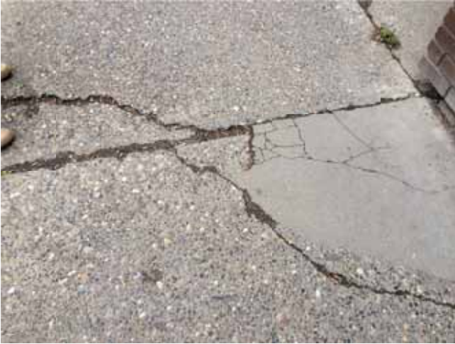
Photo 31: Cracked concrete by Reason 2 Run
