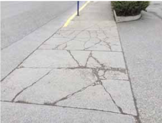
Photo 110: Cracked concrete by Chevron gas station
