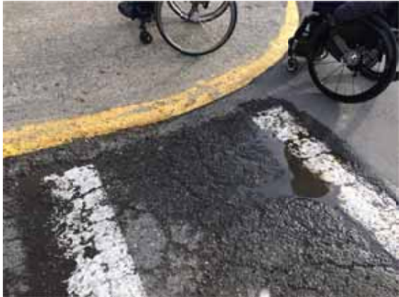
Photo 41: NE corner of Shepherd Ave and Reid St connected to crosswalk leading to NW corner – puddle, cracked asphalt, lip
