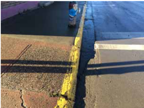
Photo 128: SW corner of Reid St. and Carson Ave -- There is no curb ramp
