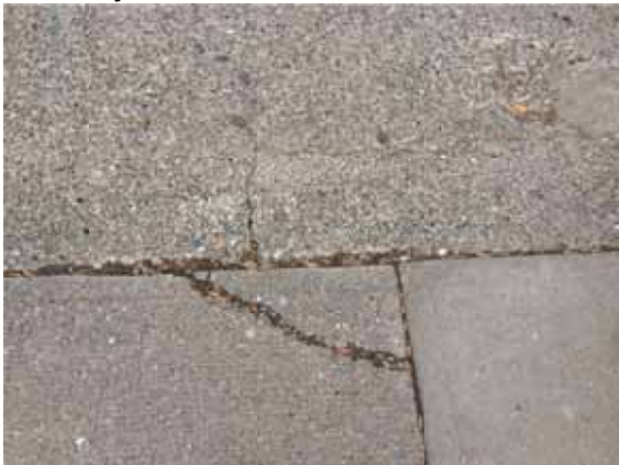
Photo 52: Cracked pavement in front of Booster juice
