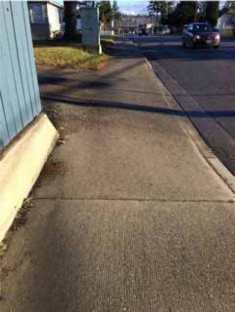
Photo 176: Lack of tactile warning in alley for people with low vision
