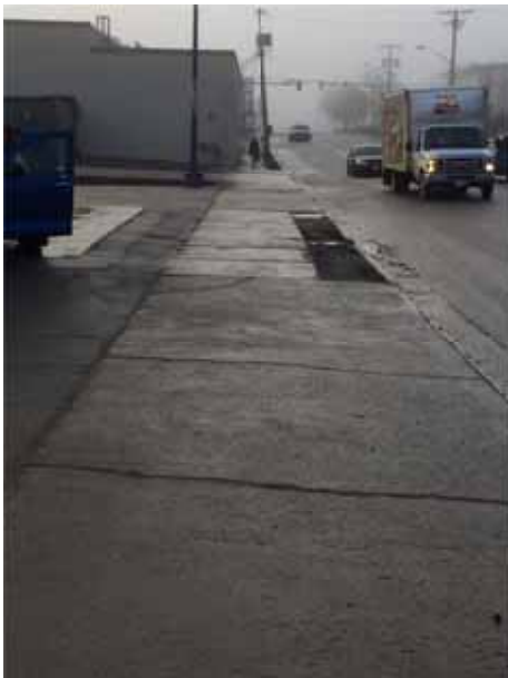
Photo 225: Looking south on the eastern side of the street – broken sidewalk sections
