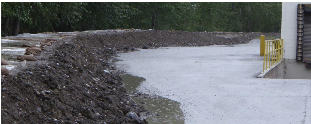
Photo 6 - 2007 – Temporary Flood Protection Along Baker Creek Near Confluence of Fraser River (Behind West Park Mall) (Source: Urban Systems Ltd.)
