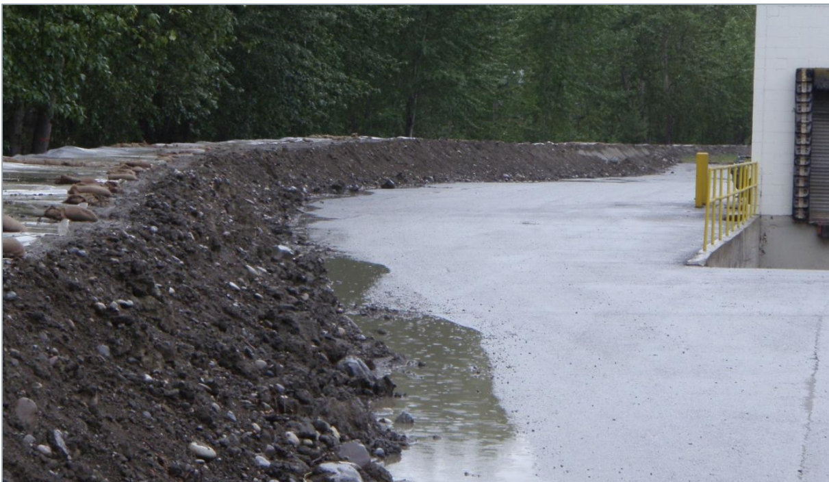
Photo 6 - 2007 – Temporary Flood Protection Along Baker Creek Near Confluence of Fraser River (Behind West Park Mall) (Source: Urban Systems Ltd.)
