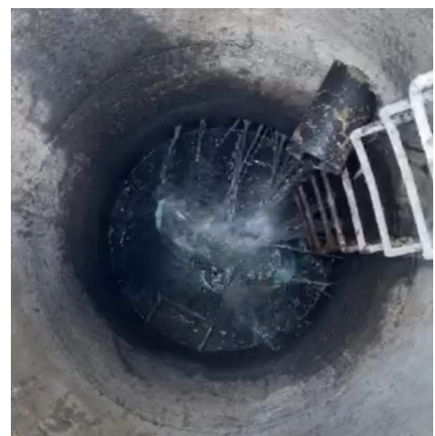
Groundwater Flowing into Manhole Behind West Park Mall (July 2020)
