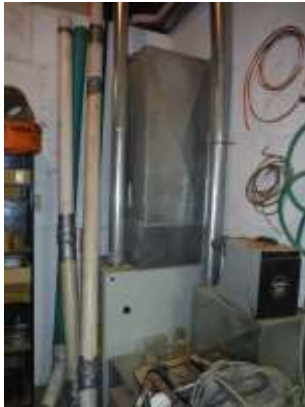
Figure 56 Furnace in Warehouse
