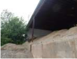
Figure 20 Bent Steel Column
