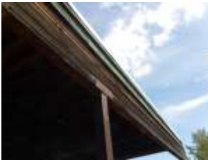
Figure 21 Damaged Glulam Beam
