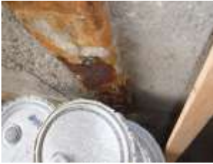
Figure 19 Corroded Steel Column
