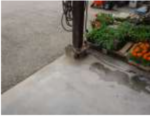
Figure 18 Pedestal Concrete Spalling
