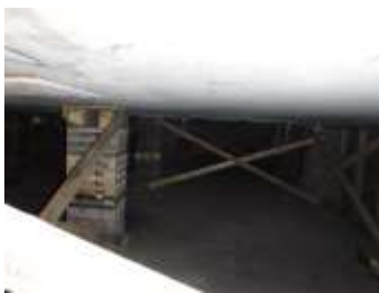
Figure 47 Wood Cribbing/Cross Bracing
