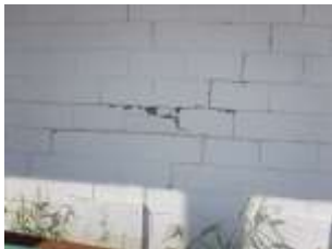
Figure 22 block wall settlement
