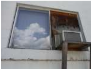
Figure 50 Old Window/AC Unit
