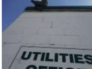
Figure 49 Block Wall Mortar Cracking
