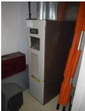
Figure 1 First Aid Station Mechanical
