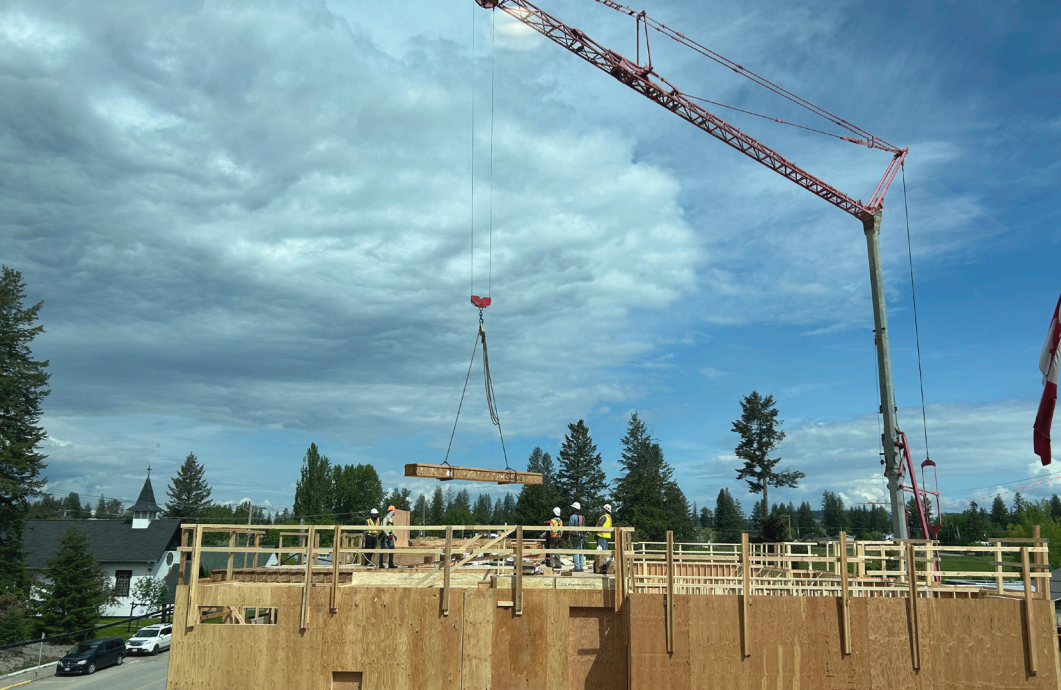
Construction of the Cosmos, a 57-unit apartment complex next to City Hall.
