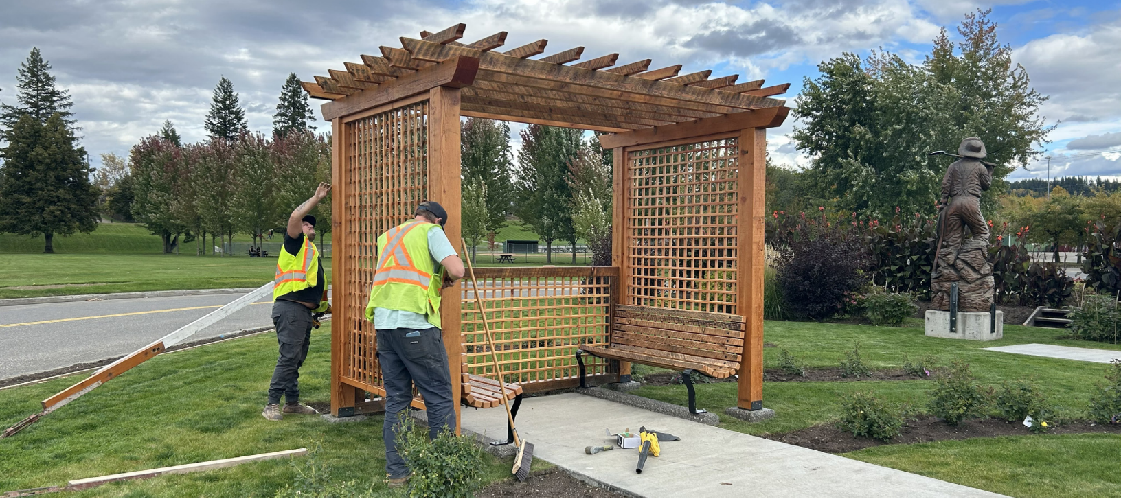
Public Works staff installing benches under the arbour in the Rose Garden.
